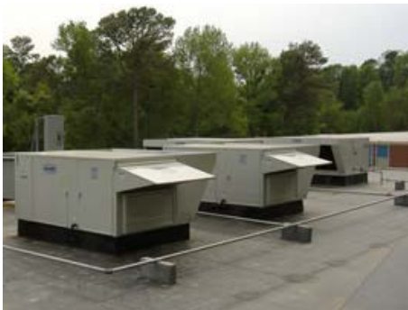
Rooftop AC Units
